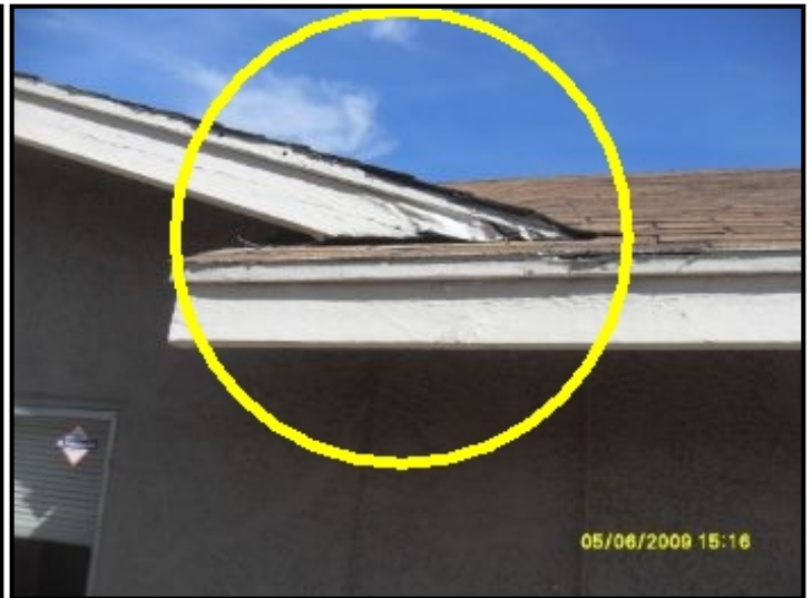
Observed separation/deterioration of fascia
