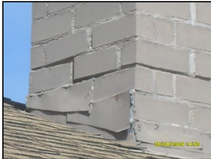
Some mortar deterioration observed; advise repair as needed.
