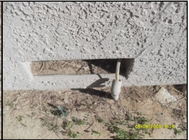
Observed wires coming from garage vent. unknown. this needs to be checked for use of wires by a licensed electrician
