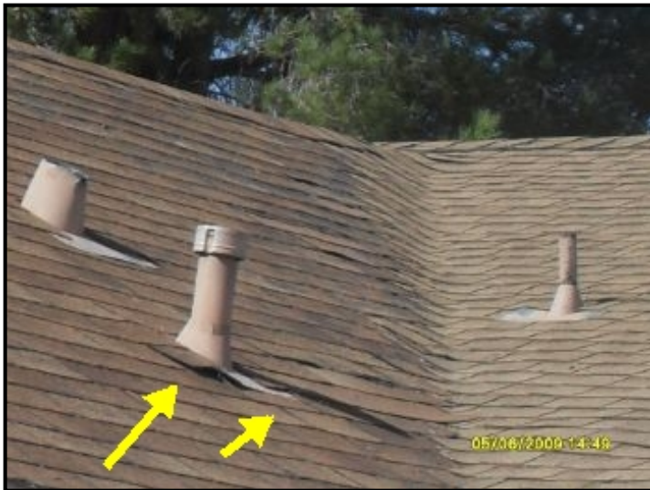
Observed curling tile at penetration
