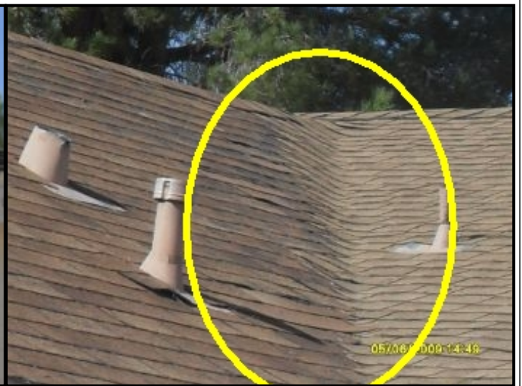
Appears to have been prior repairs
