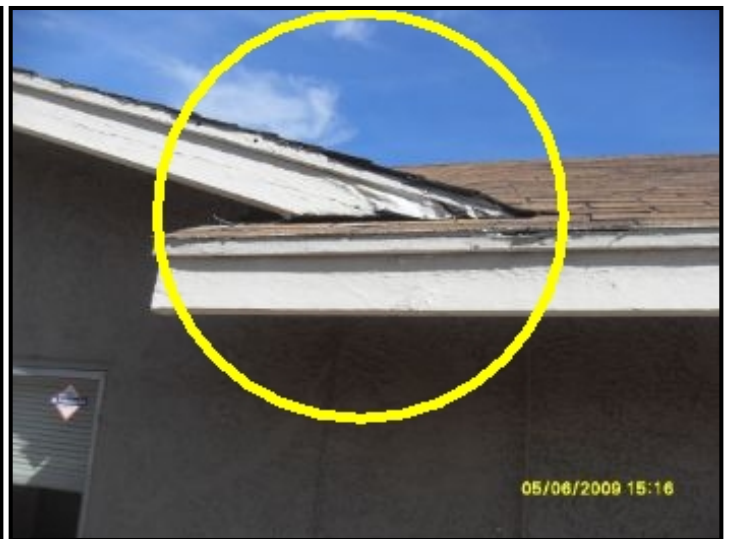
Observed separation/deterioration of fascia
