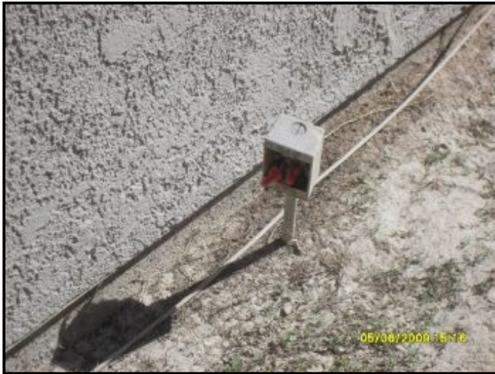
Junction box missing cover plate
