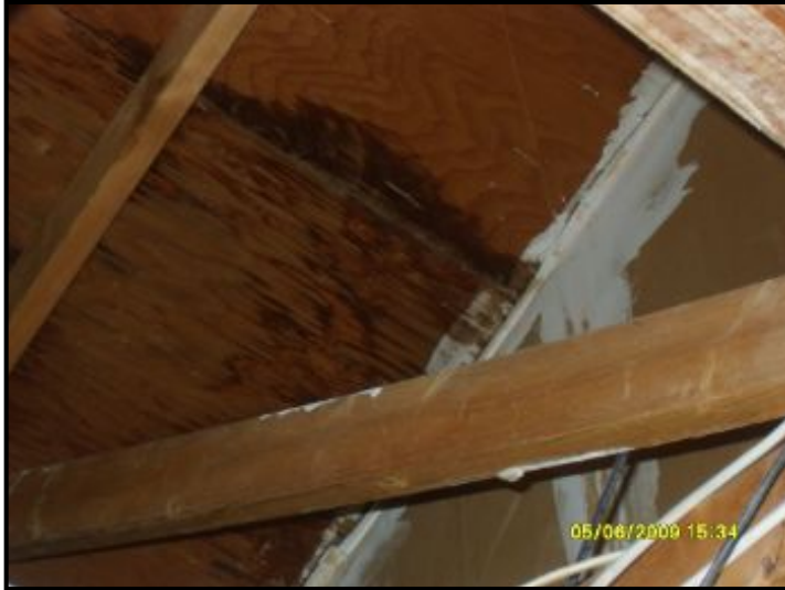
Observed prior stain on ceiling and wall
