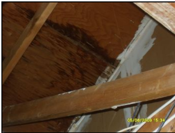
Observed prior stain on ceiling and wall
