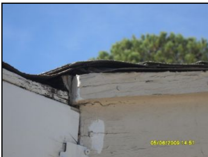
Visible deterioration was noted.
