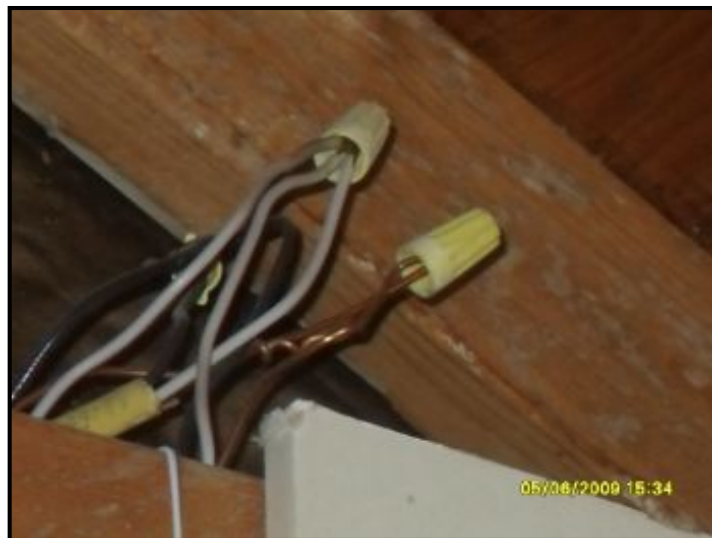
Recommend full review by qualified electrical contractor
