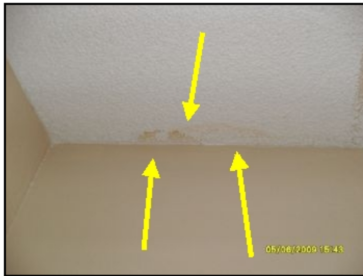
Noted stain on closet ceiling
