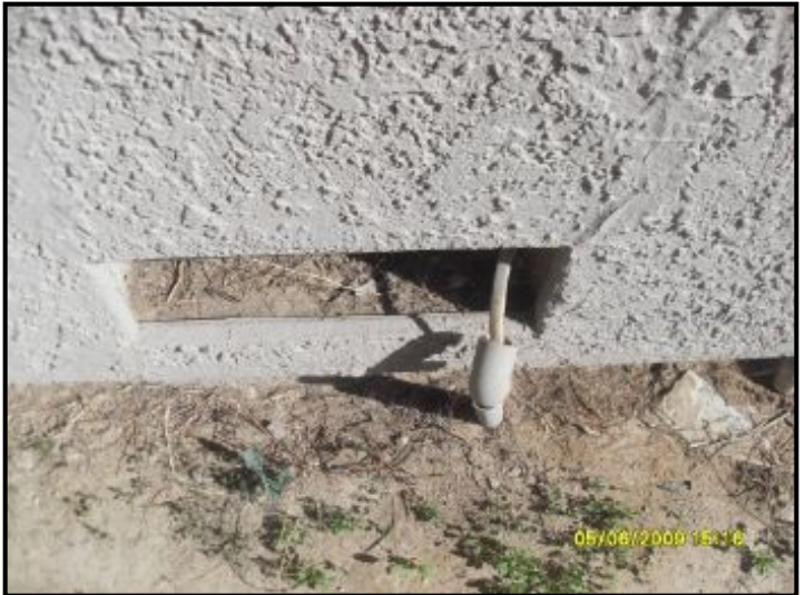
Observed wires coming from garage vent. unknown. this needs to be checked for use of wires by a licensed electrician
