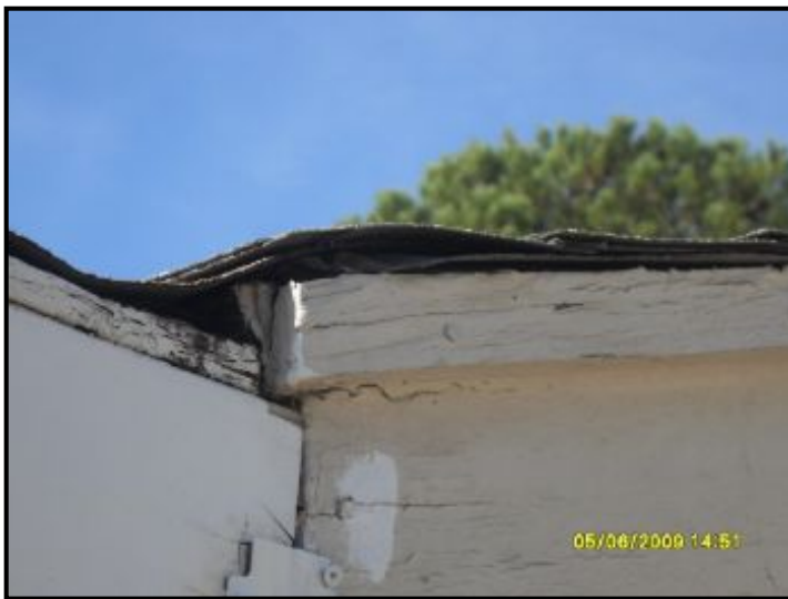
Visible deterioration was noted.
