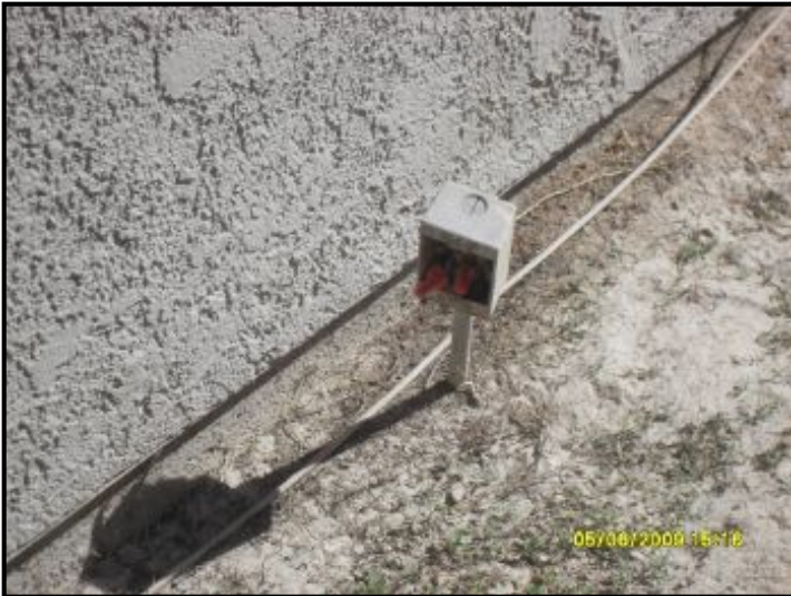
Junction box missing cover plate
