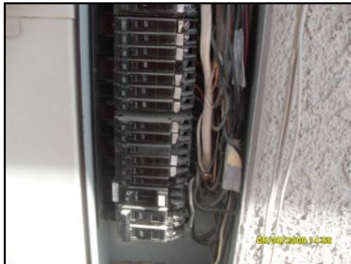
When panel cover off there is a lot of wires in box which obstructs a full inspection of the main panel
