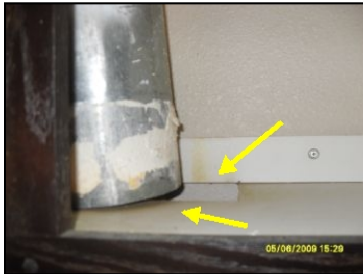
Observed air leaking from duct when exhaust fan operated, this should be sealed to allow exhaust to vent to the exterior
