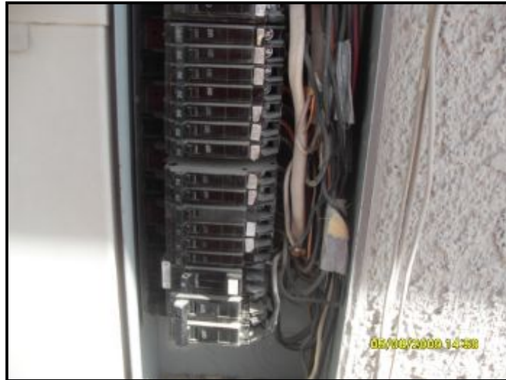
When panel cover off there is a lot of wires in box which obstructs a full inspection of the main panel
