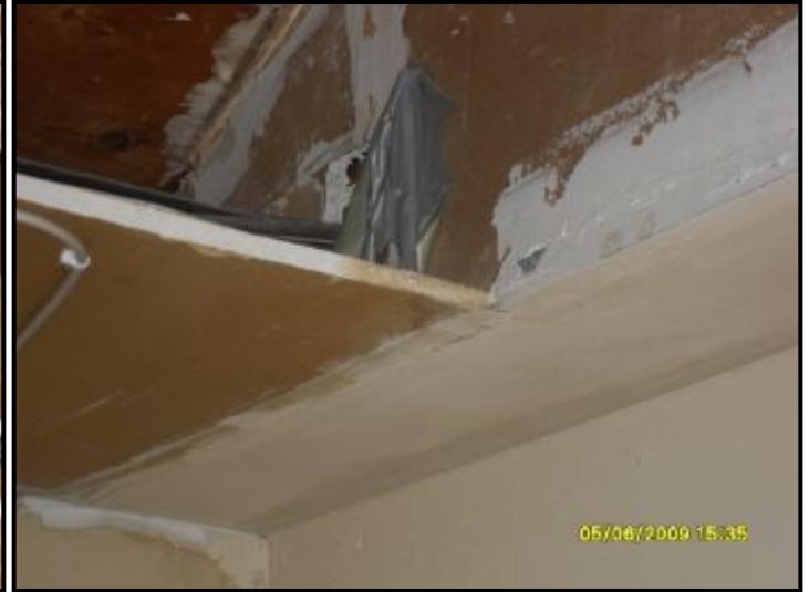
Fire wall between garage & house needs repair for fire standards
