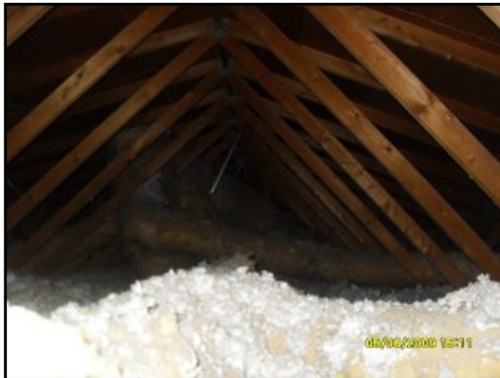
This type of insulation obstructs a visual inspection of many areas in attic
